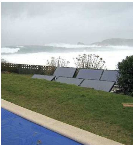
Solar thermal energy installation covering a total capturing surface of 12 m 2 for sanitary hot water and swimming pool heating in Meirás (Valdoviño)
