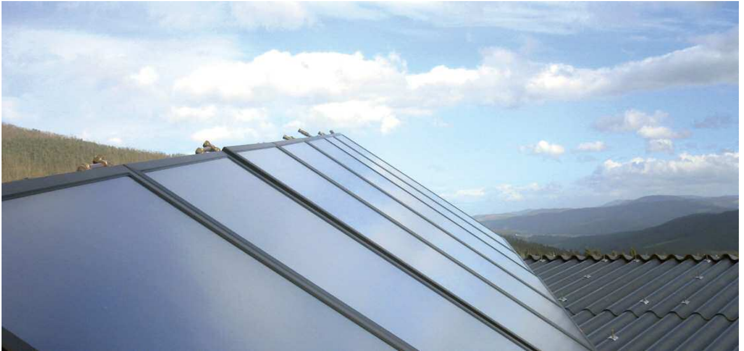
Solar thermal energy installation covering a total capturing surface of 32 m 2 for sanitary hot water in Ribadeo (Lugo)
