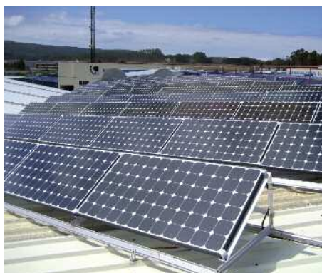
23.52 kW on a warehouse roof in Narón (A Coruña)
