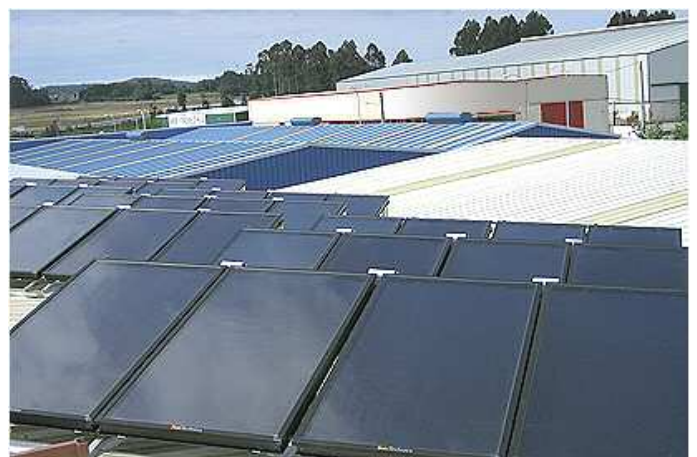
Installation with a capturing surface of 96 m 2 for solar air conditioning with absorption machines in Narón (A Coruña)
